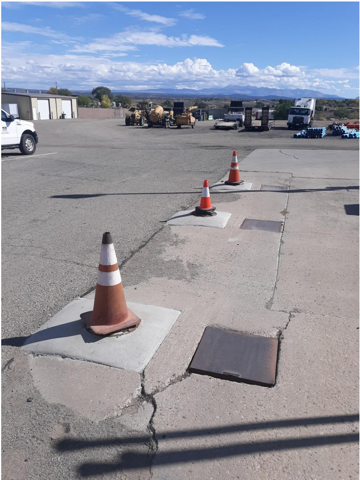
Upper Yard Underground Tanks Fuel Fill Ports (To Be Removed)
