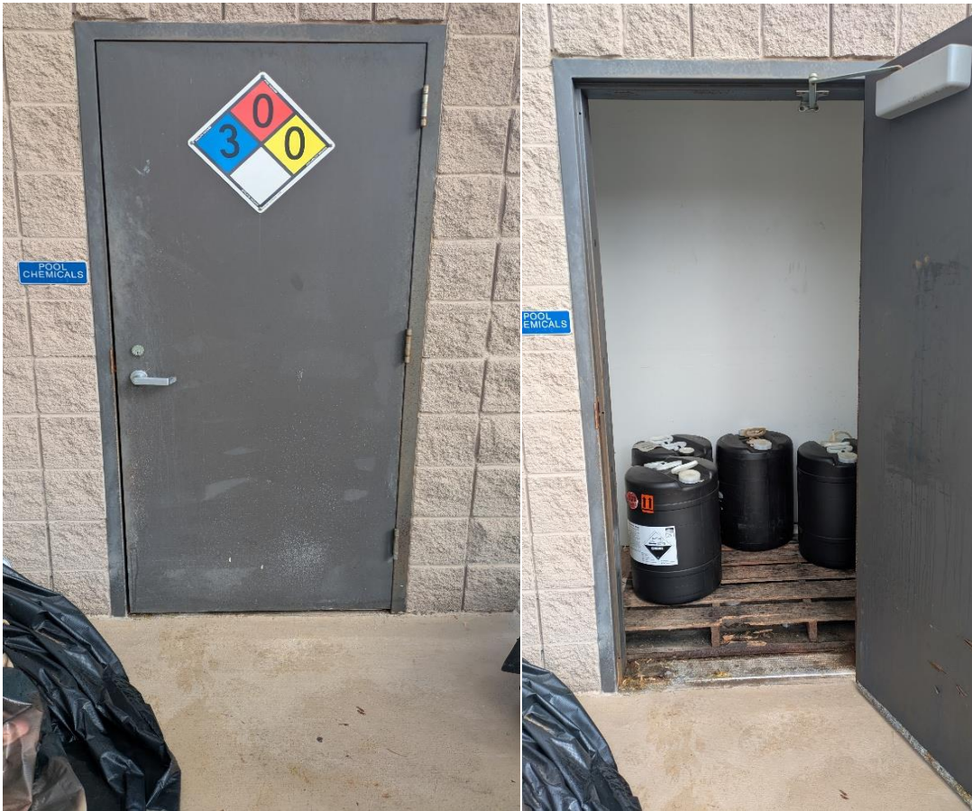
Pictures 1 and 2 – Door to be replaced.
