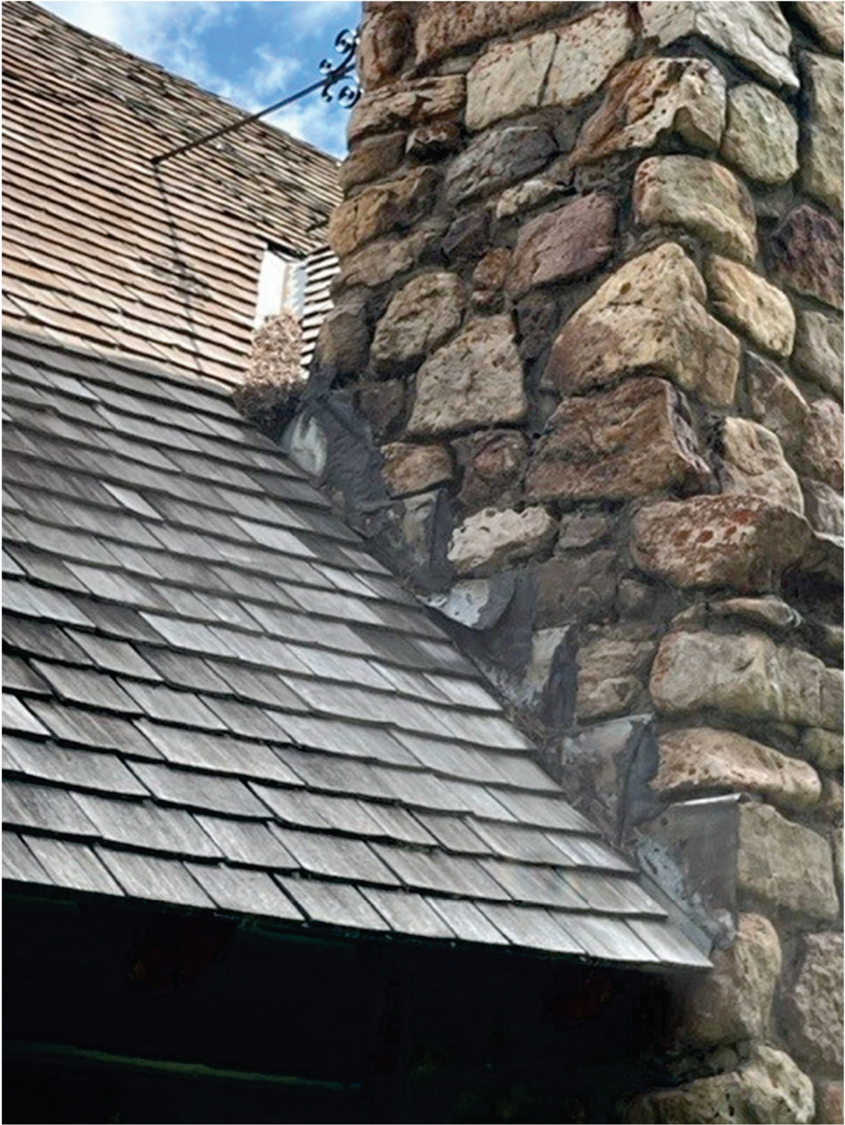
West Chimney Flashing and Masonry
