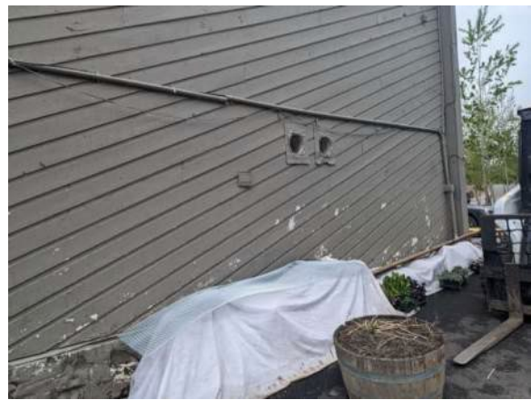
Photo #21 Uncovered vents on North elevation of Maintenance Building – also cover for rodents up against
