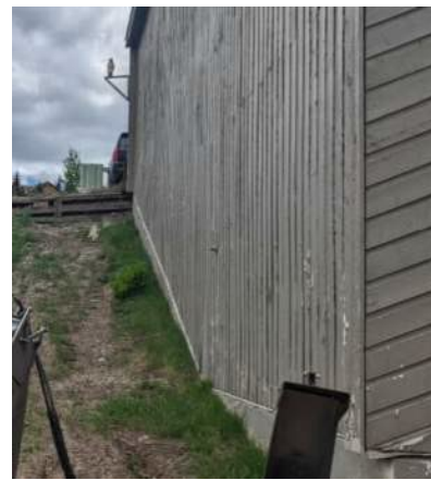
Photo #22 Gaps in cladding on east elevation of Maintenance Building
