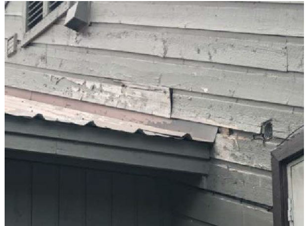
Photo #20 Gaps in cladding that exceed \frac{1}{4} inch, Town Hall building
