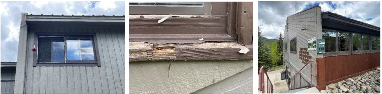
Photo 11, 12 and 13 (Left to Right): North-facing Town Hall building elevation with existing wood-framed horizontal slider window (note deteriorated wood siding beneath roof cap flashing); severely deteriorated wood sill plate and paint below window assembly; overview of south-facing building elevation, with metal-framed horizontal slider windows (at right).
