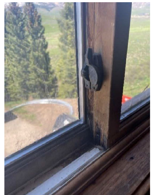
Photo 22: Stain at interior of existing wood window frame, within Town apartment unit.
