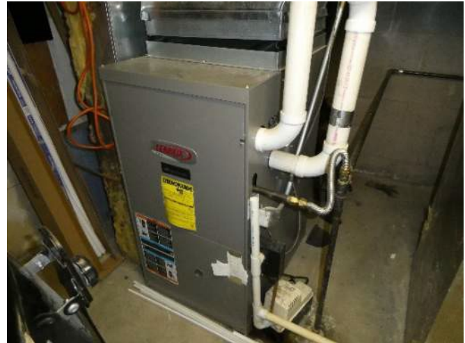
Photo 20: Overview of Town Hall Building mechanical equipment and piping connections within first floor mechanical room.
