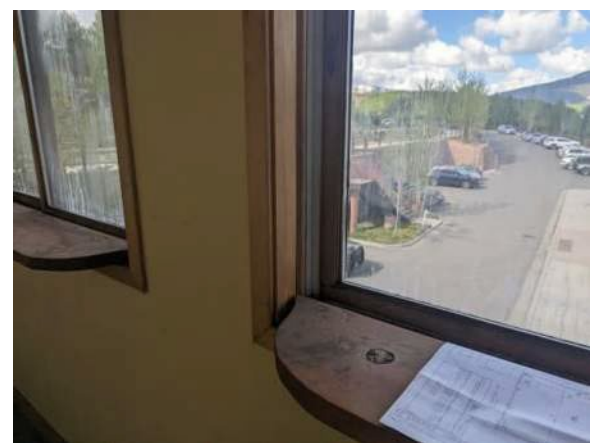
Photo #24 Evidence of condensation on windows on top floor of Maintenance Building
