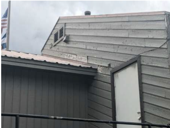
Photo #19 Vents with greater than \frac{1}{4} gaps on Town Hall Building
