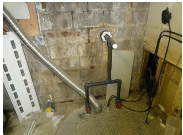
Photo 22: Domestic water main shutoff valve and meter within first floor mechanical room of Town Hall Building.
