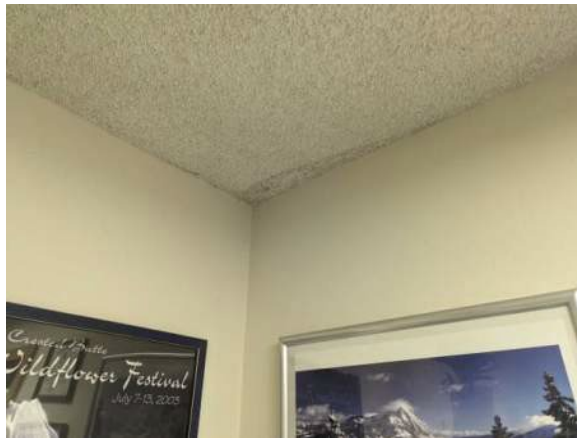
Photo #15 Evidence of prior roof leak in one of the offices in Town Hall Building
