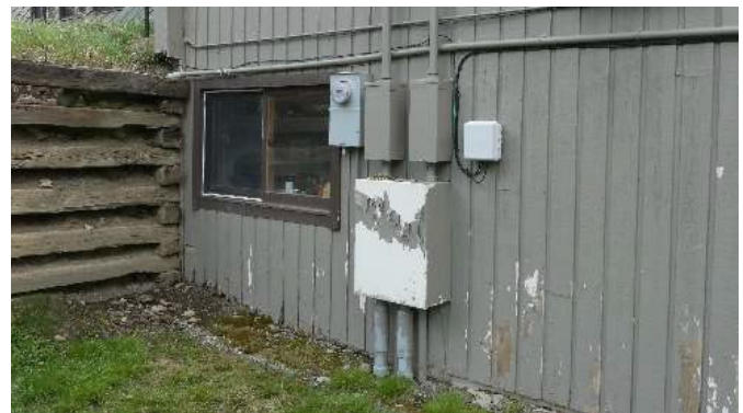
Photo 21: Overview of Town Hall Building electrical service disconnects located on the north exterior wall.
