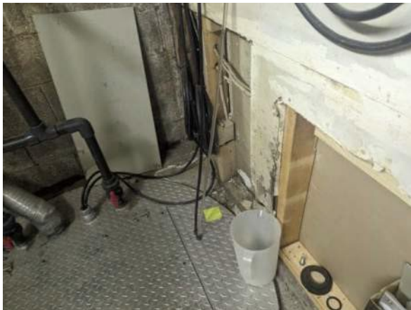
Photo #11 Small amounts of visible mold growth on drywall paper in the mechanical room of Town Hall Building
