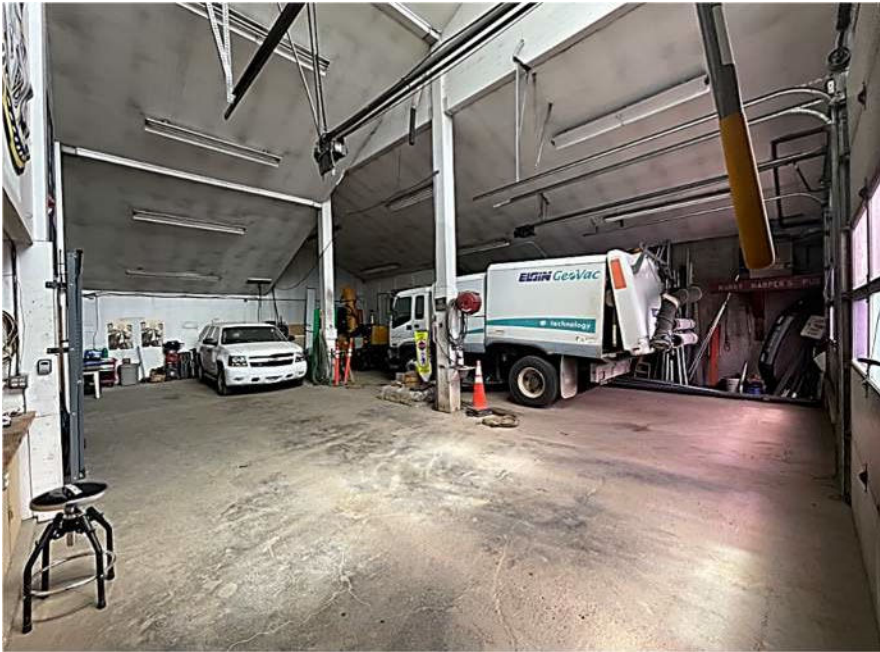
Photo 28: Overview, including visible slab cracks, at upper garage bay of Town Maintenance Facility.
