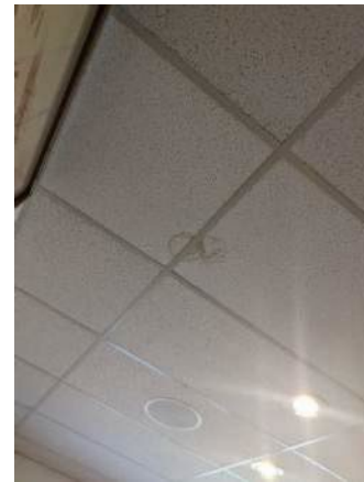
Photo #16 Evidence of prior roof leak in the town council chambers, Town Hall Building
