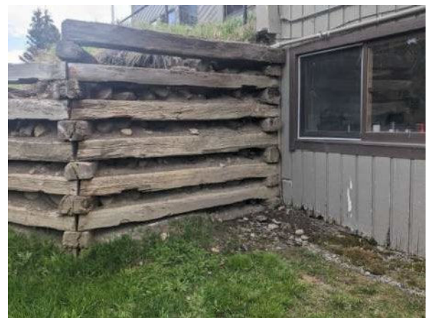
Photo #18 Gaps greater than 1/4 inch along the bottom of the wall – Town Hall Building
