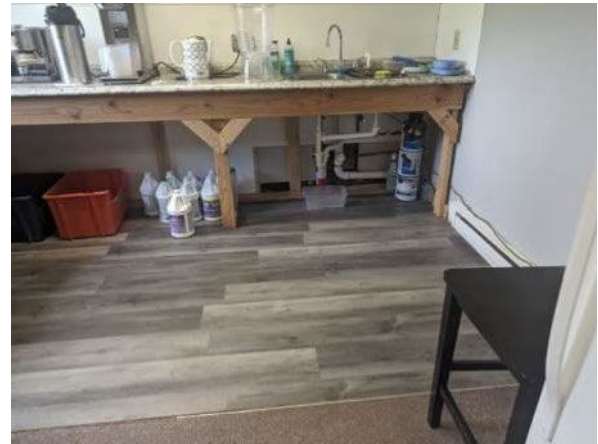
Photo #14 Breakroom wall that was remediated for mold following a roof/water infiltration event
