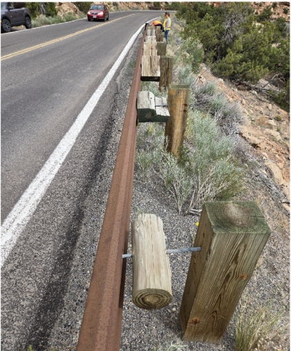
Example of Damaged Blockouts
